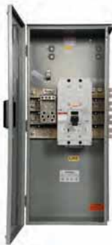
Main Circuit Breaker
