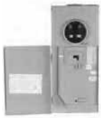
Meter Breaker with Interlock Cover
