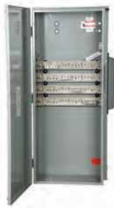
Main Terminal Box
