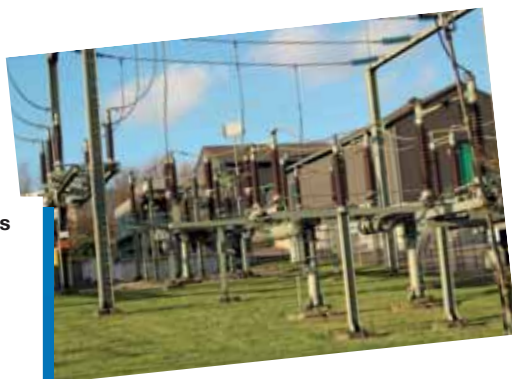
Aluminum compression cable lugs are frequently used in power distribution.
