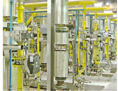
Walking beam furnace with overhead firing
